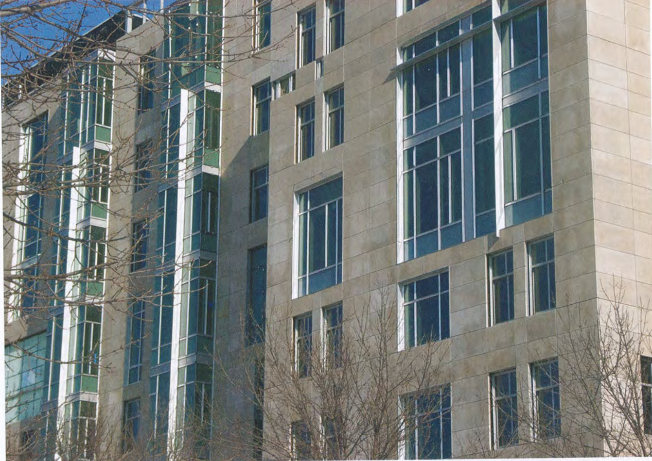
Use of a rain-screen system not only saved money on construction, but reduces future maintenance because the joints aren't sealed. (Photo courtesy Goody Clancy)
