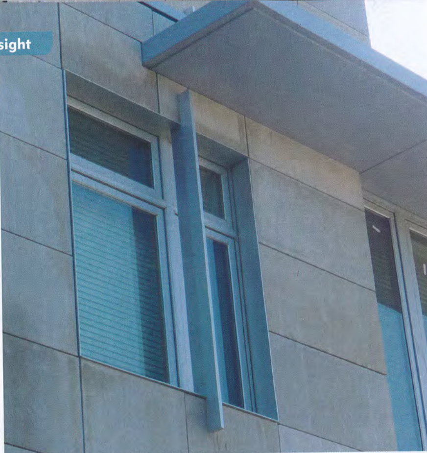
The variety of stone sizes used in the project is apparent at the top of the photo. Some pieces were so small that installing four anchors became a problem. (Photo courtesy Goody Clancy)
