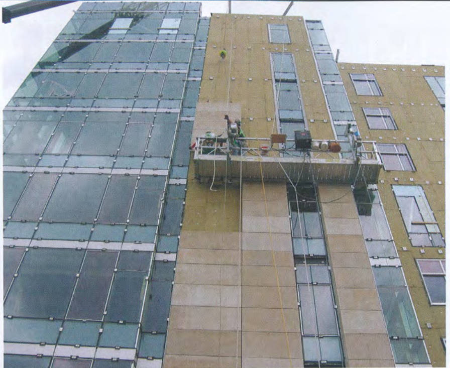
The first unitized panels go up on the building. It's also readily apparent that not all the stones – and panels – are the same size. (Photo courtesy ASI Limited)
