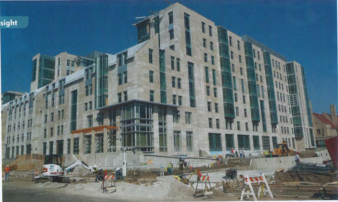
A wide-angle shot displays the sheer size of the new hall, which currently holds more than 800 residents. Set on the edge of the campus, the nearness to the adjoining neighborhood is evidenced by the home in the background at far right. (Photo courtesy Goody Clancy)
