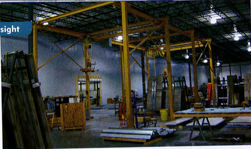
ASI had to install new equipment and learn new processes to get the University of Chicago job. The panels had their own assembly area within the company's Whitestown, Ind., plant. (Photo courtesy ASI Limited)
